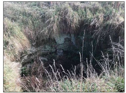
Photo 18: Drainage sump on east stretch of trotting track
