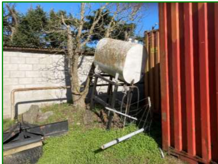
Photo 7: Diesel AST on sloping ground
