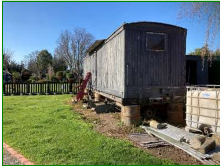
Photo 6: Railway carriage with flaking paint
