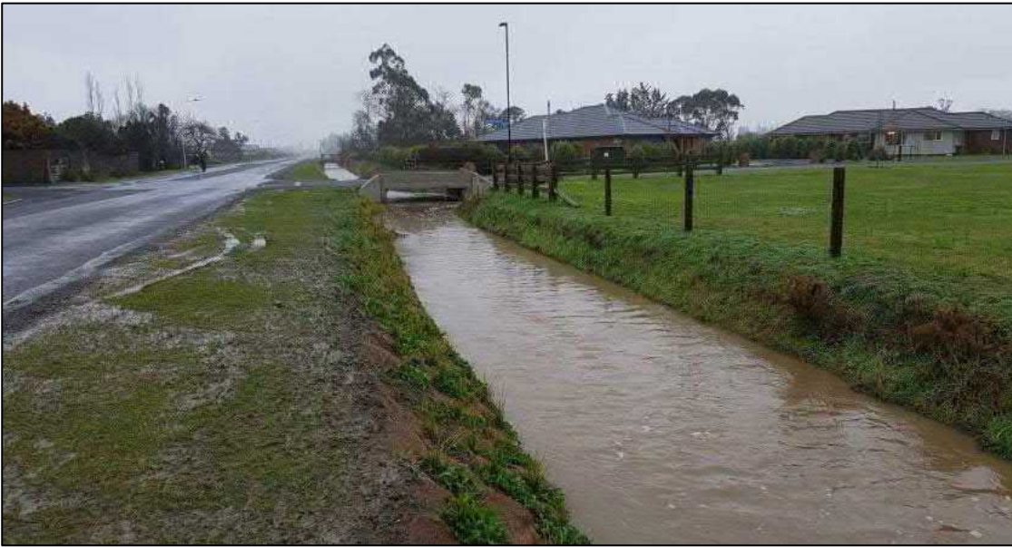
Photo 3: Upgraded Manse Road Drain during a higher rainfall event. Looking north from High Street.
