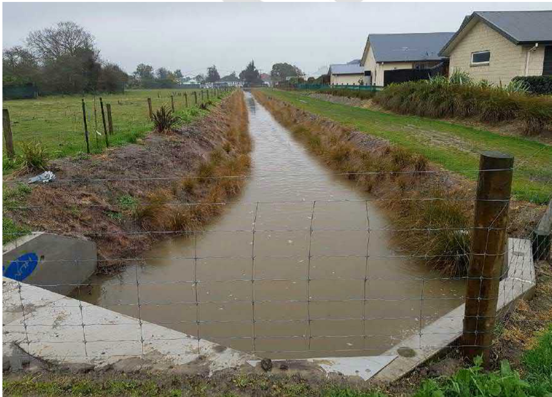
Image 4: Upgraded CDHB Drain in Flood
