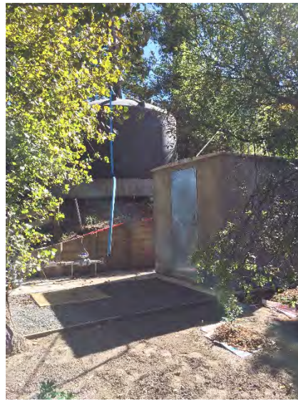
Photo 2: Reservoir and booster pump shed
