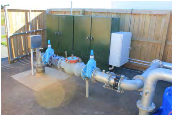
Photo 3: Elizabeth Allen Drive Wellhead
