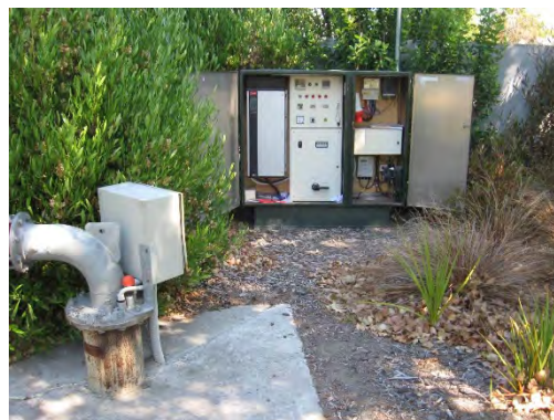
Photo 4: St Patricks bore and control cabinets
