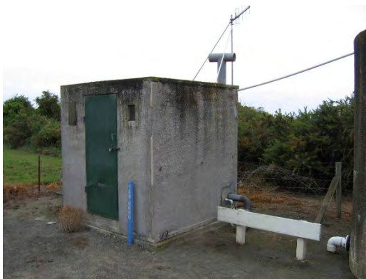
Photo 1: Pump Shed and reservoir
