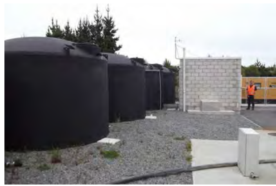
Photo 2: Rossington Drive Tanks and Pump Building
