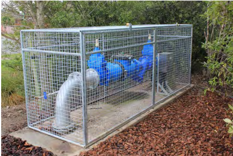
Photo 1: Gallipoli Street Well Head
