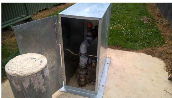
Photo 1: Well and pump shed
