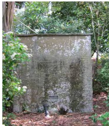
Photo 2: Millstream pump shed
