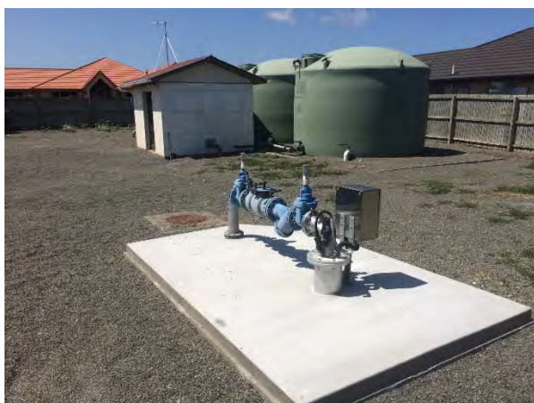
Photo 1: Bore headworks and reservoirs
