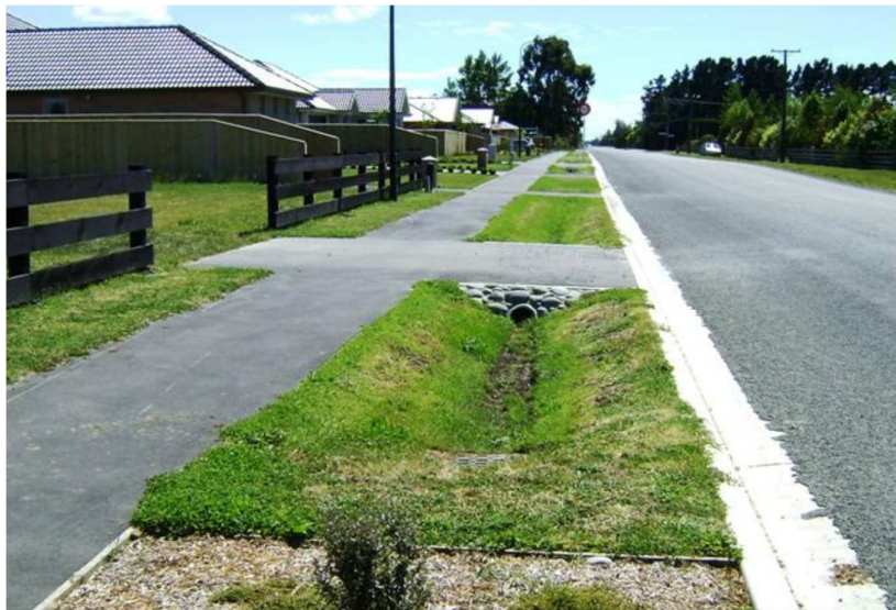
Figure 9.1.3: Treatment Swale — Brookside Road
